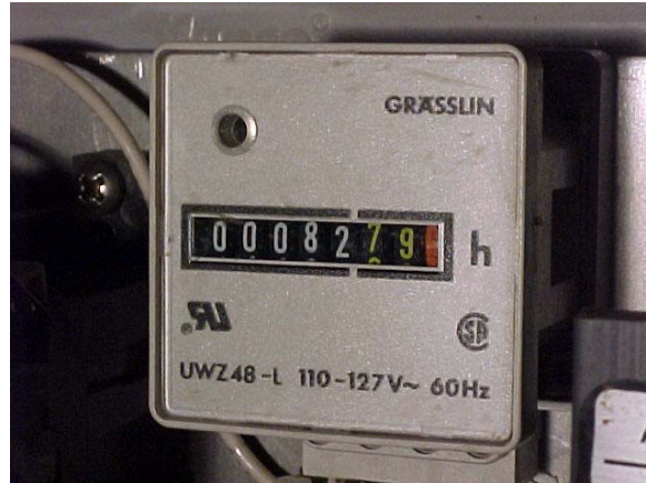
Figure 6: Elapsed Time Meter
