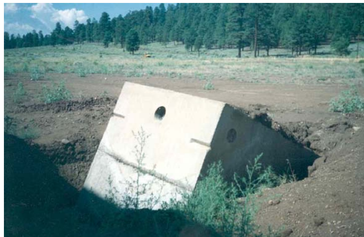
Figure 17 Septic Tank Dislodged By Buoyancy Force
